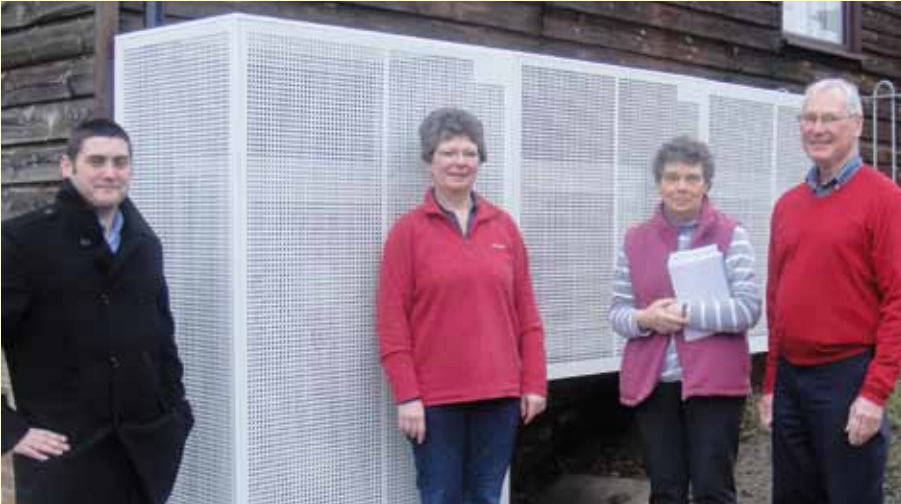
Pictured are Dan Wood of Acrol, with committee members Teresa Scott, Vera Filer and Brian Talkes, by the security cages that protect the heat pumps on the outside of the building
